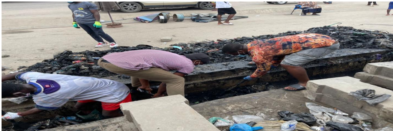
Figure 5: Desilting of a public drain along the Kasoa Bawjiase Road on 25th October, 2025
