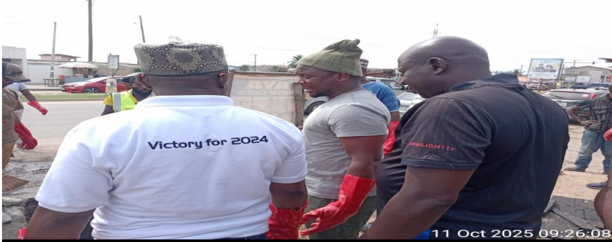
silting of public drain around the Obom road to ensure the free flow of waste water during the Sanitation Day Celebration on the 11 th October, 2025.
