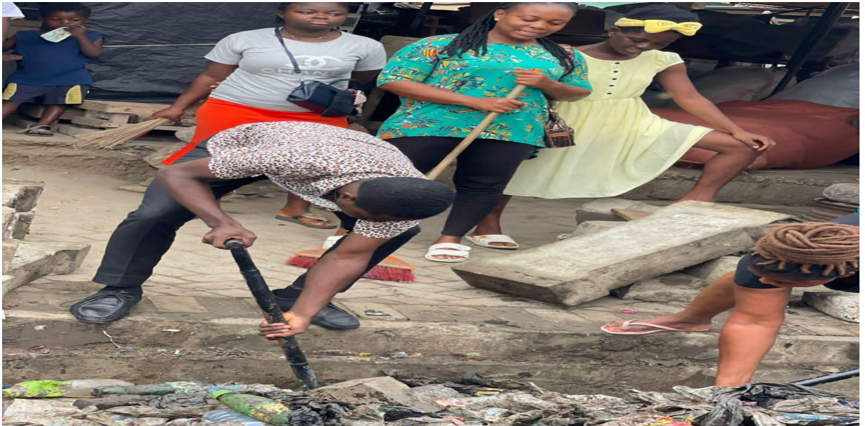
Figure 5: Desilting of a public drain along the Kasoa Bawjiase Road on 21st September, 2025
